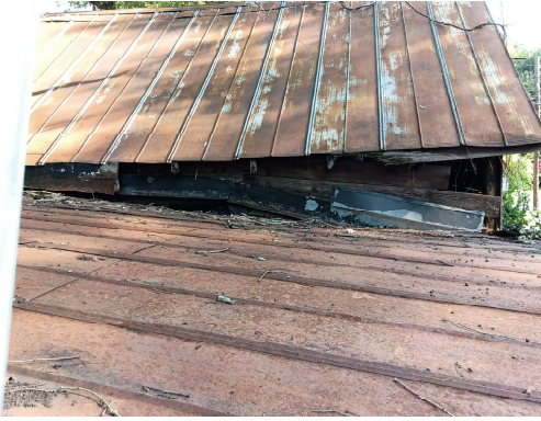
Siding failure that caused framing damage
