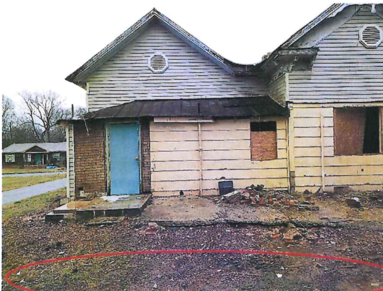
Back driveway was gravel. Soil incursion and lack of maintenance.
