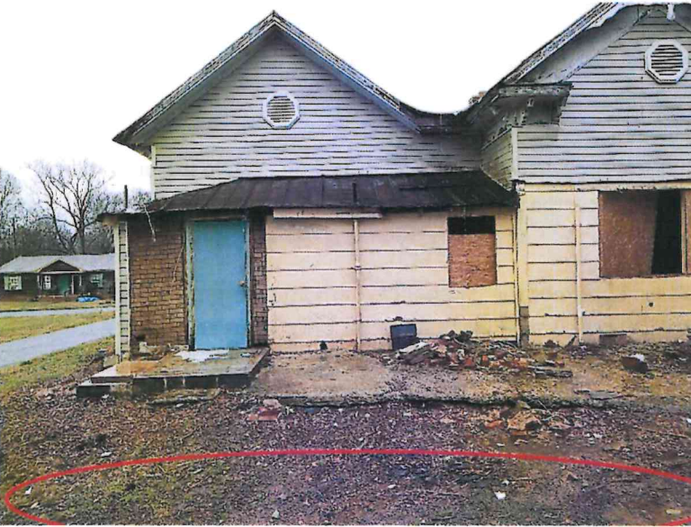
Back driveway was gravel. Soil incursion and lack of maintenance.
