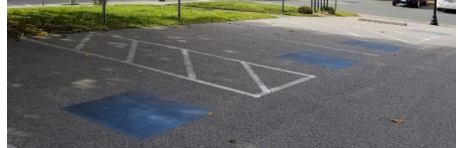
Image 10 – Worn striping and stencils – Police Station Lot
