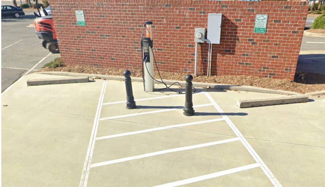
Image 7 - EV Charging Station - Correll St. Parking Garden
