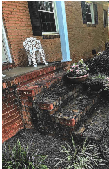
Existing front porch without rails
