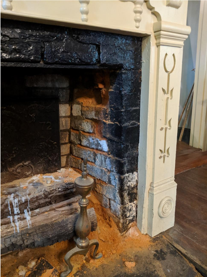
Interior Photo of Chimney, brick deteriorating.
