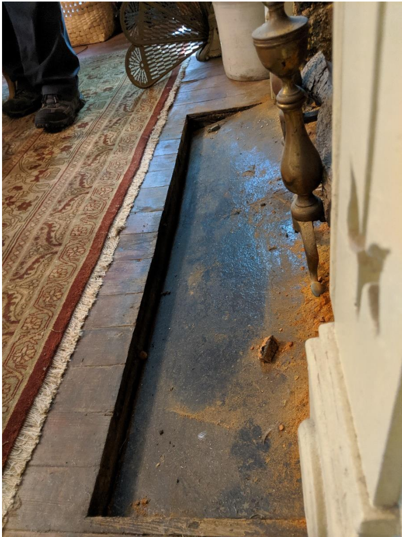
Hearth of fire place damaged
