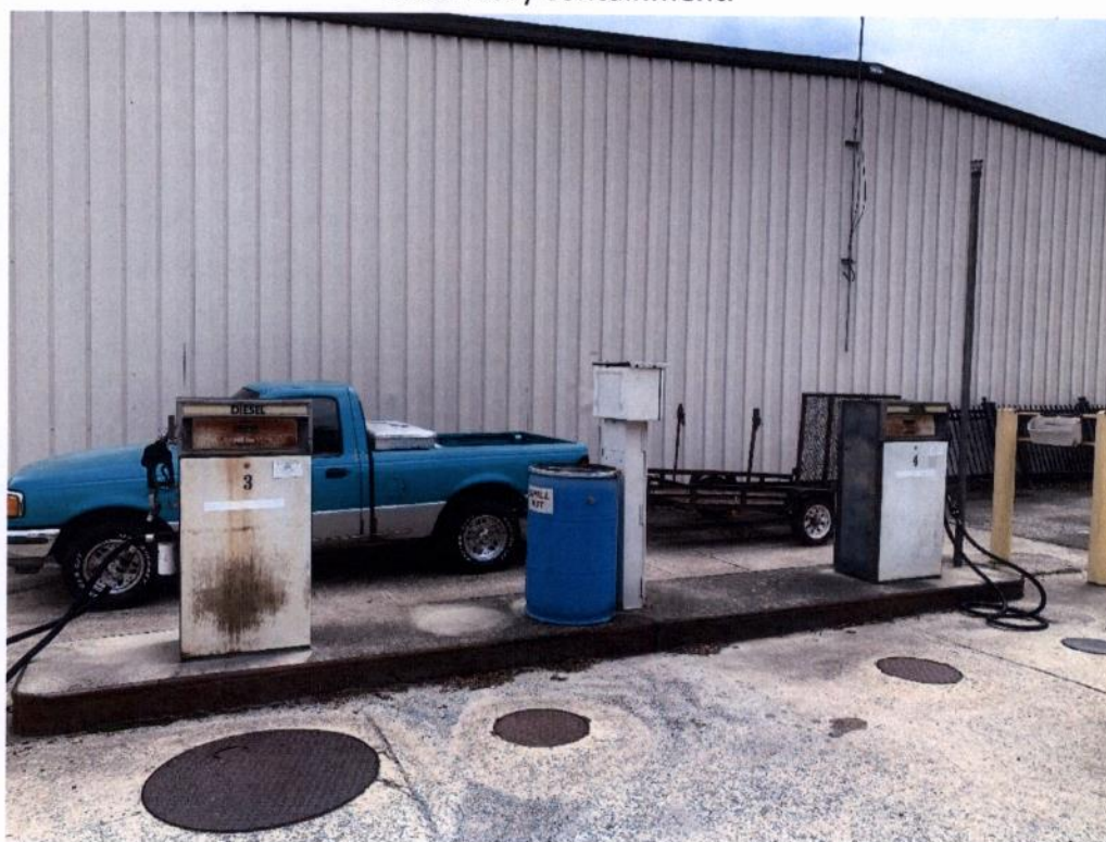
Photograph 8: View of fuel island at Facilities Maintenance.
