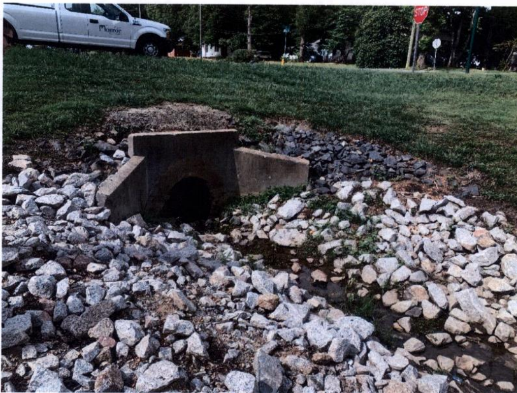
Photograph 10: View of outfall number 2812.
