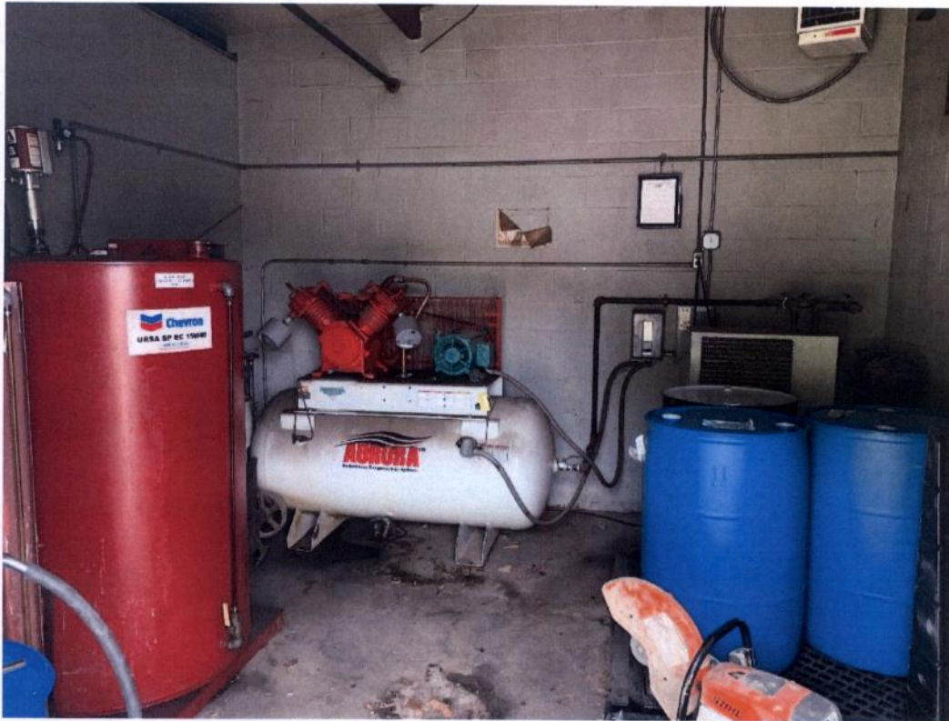
Photograph 3: View of bulk oil and hydraulic fluid storage at the Operation Center.
