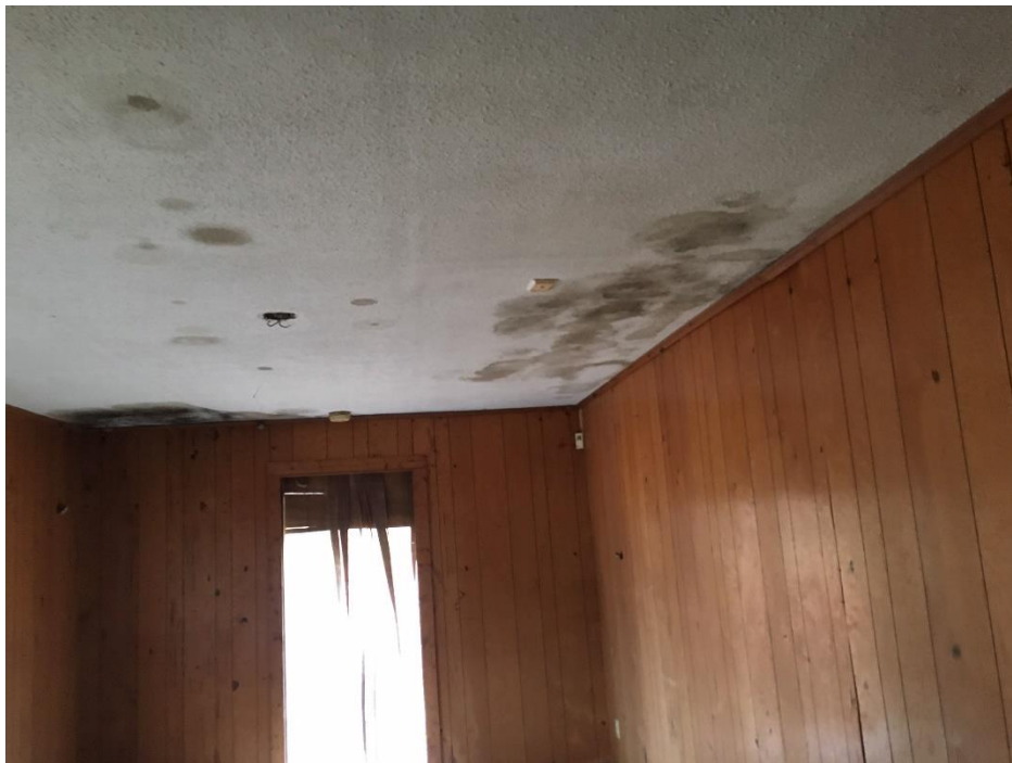
Photo 20 Interior of abandoned structure located on Parcel 09-301-226B
