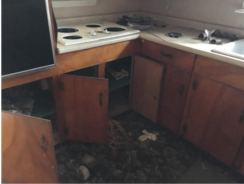
Photo 19 Interior of abandoned structure located on Parcel 09-301-226B
