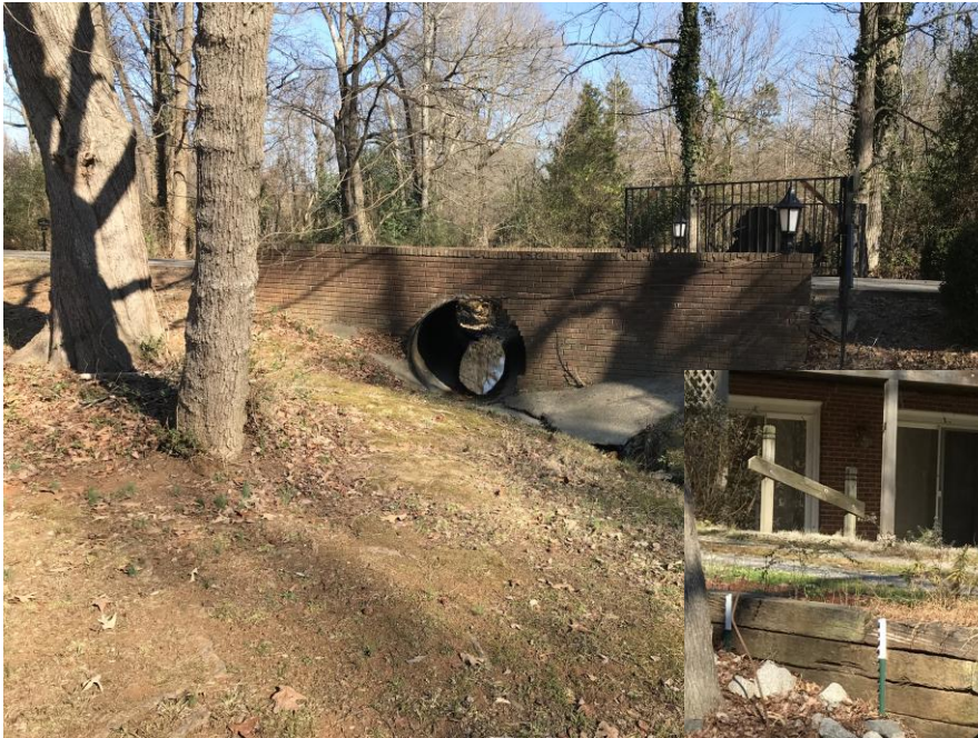
Driveway pipe at 2209 Melody Drive
